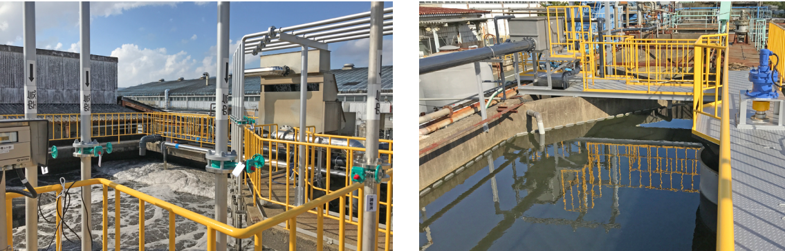
Wastewater treatment equipment at Business Site 2 in Japan
