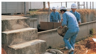
Kyushu Sekisui Ind., Co., Ltd. Sand bag piling to minimize expansion of contamination
