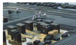
Rainwater storage tanks
