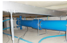
Drinking water storage system
