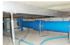
Drinking water storage system
