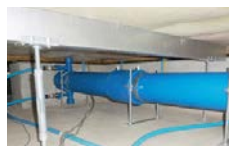
Drinking water storage system
