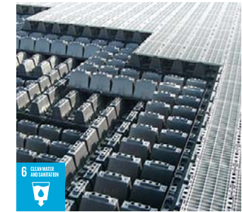
Rainwater storage system
